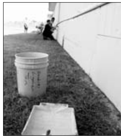
Soldiers of the 263rd Maint. Co., 553rd CSSB, 4th Sust. Bde., 13th ESC, help paint the walls outside the Success Lab at Midway High School's alternate education center June 26.
